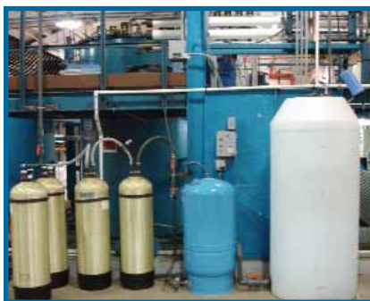
Master Metal's high-tech water filtration system generates rinses that exceed some aerospace specifications two to four times over.
